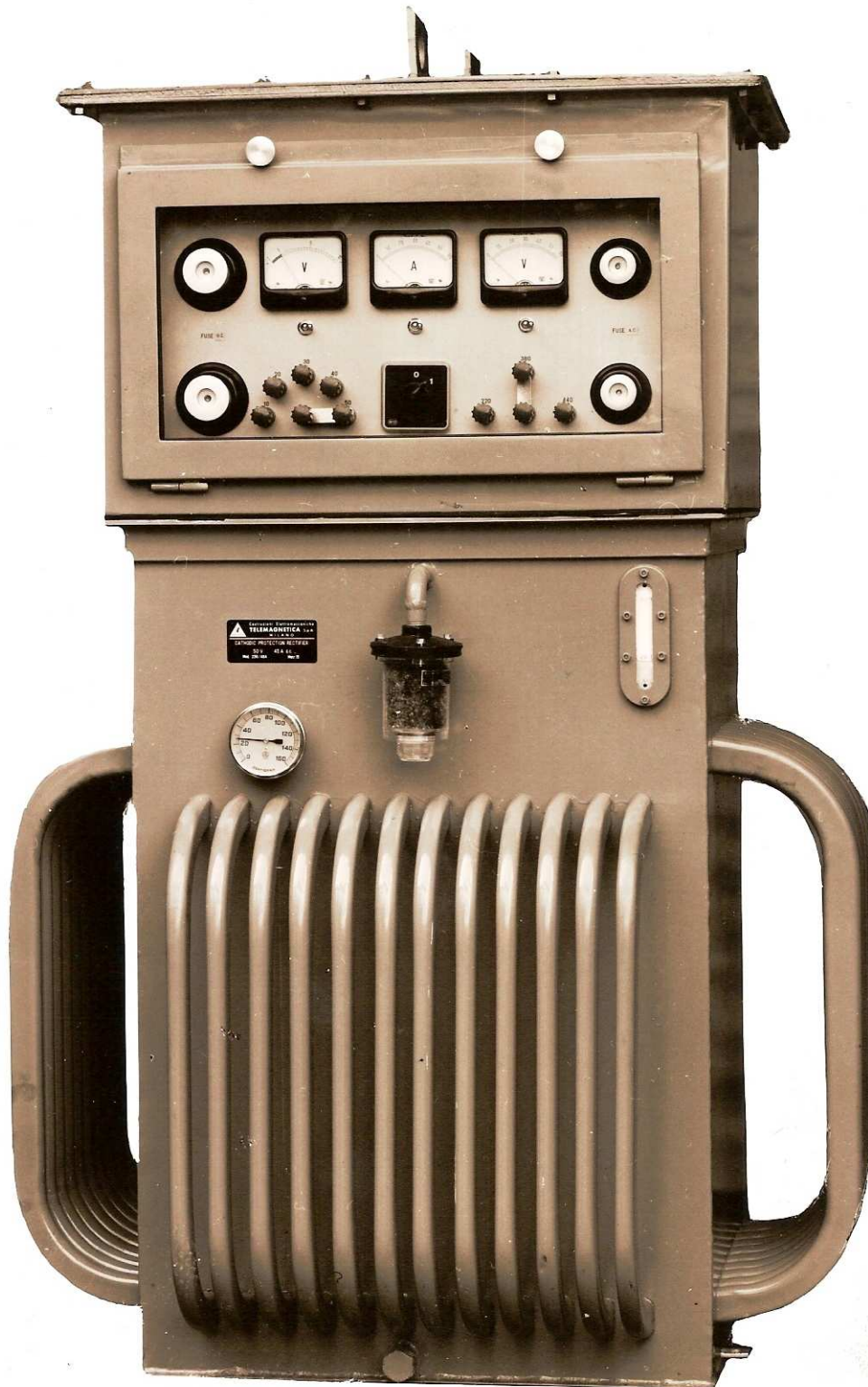
Transformer rectifier oil cooled mod. 236-48°
